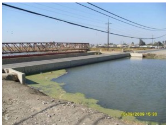
The Russell Avenue bridge once passed more than 2 feet above the water, but it has been sinking as a result of groundwater pumping and now is nearly submerged in the canal. US Geological Survey
