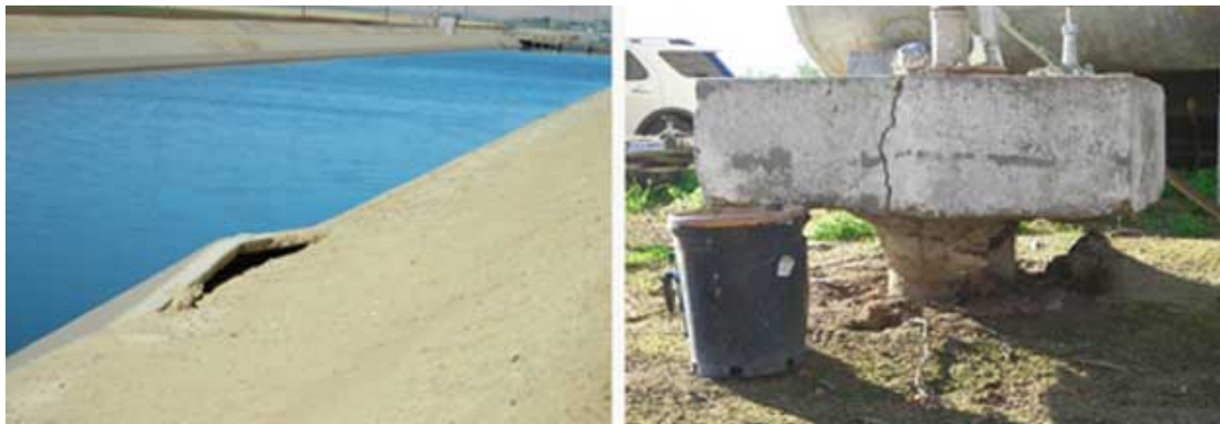
The wall of a canal (left) cracks as the earth around it sinks. The top of a well (right) is pushed up and out of the ground as the ground around it sinks. US Geological Survey
